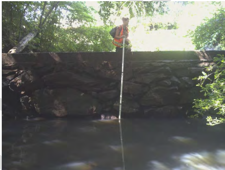
HVA Staff measuring Deep Brook Dam and facing the downstream wall of dam
