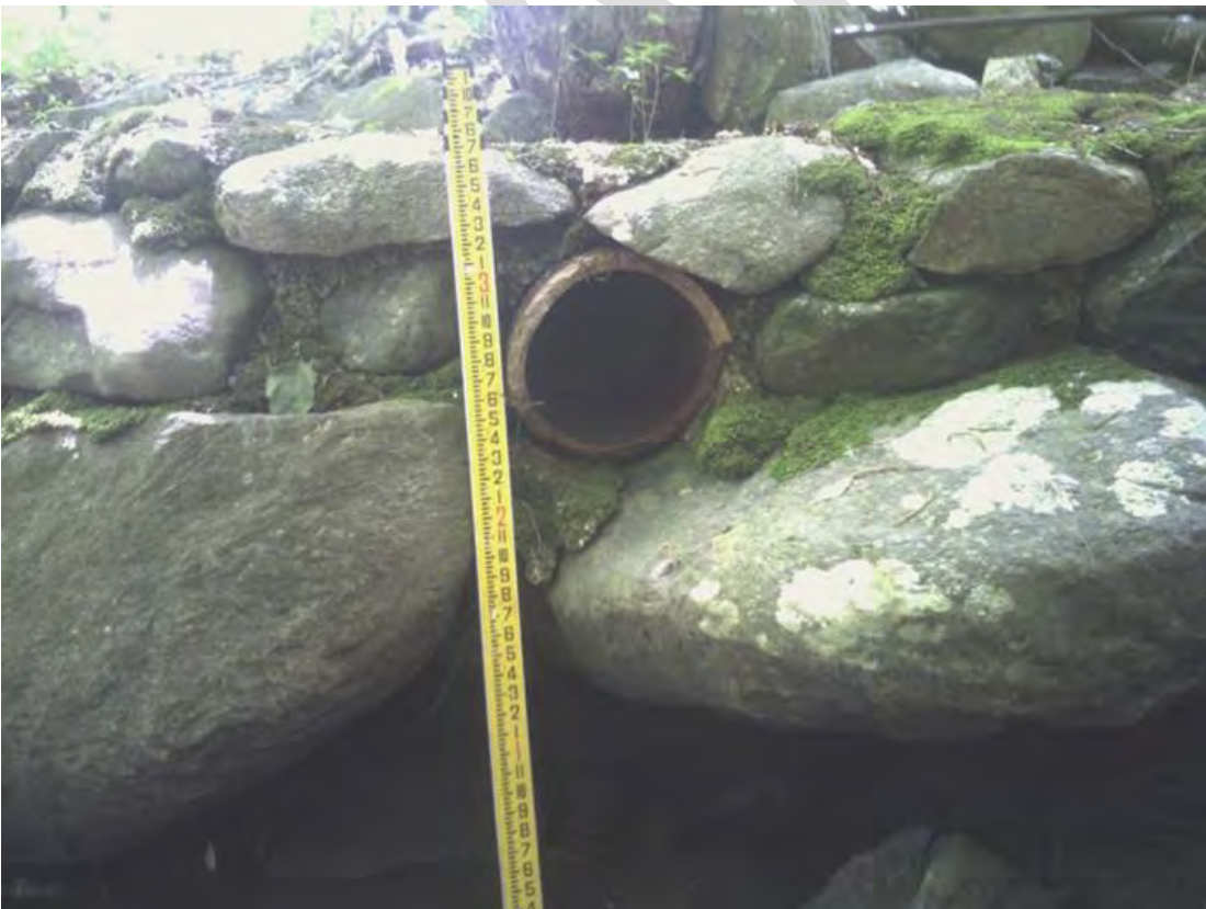
Stormwater outfalls into Deep Brook. Suspected connections to CT DOT Highway Garage.
